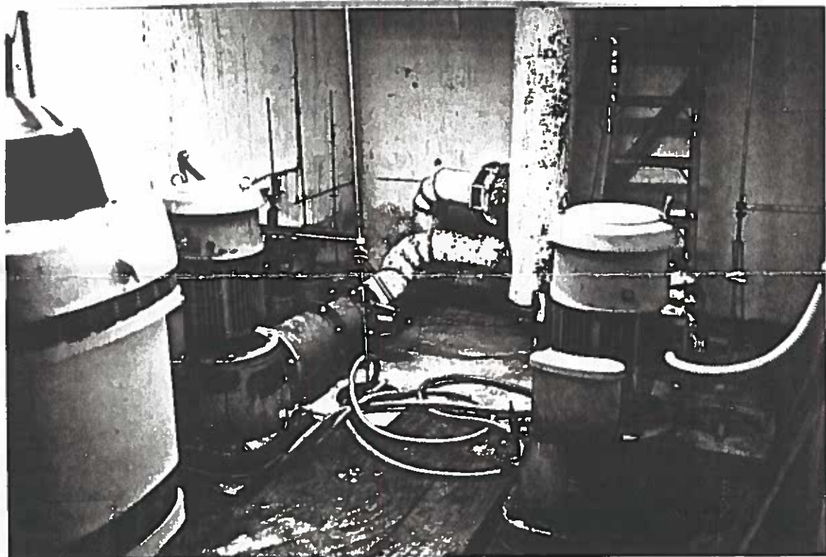
Inside of shed with distribution pumps
