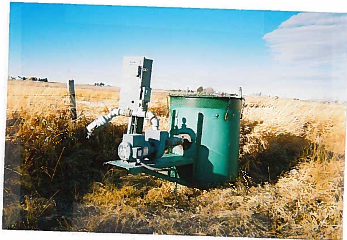
Percin stand pipe \frac{1}{2} 5 hp. pump on Great Western Canal.
