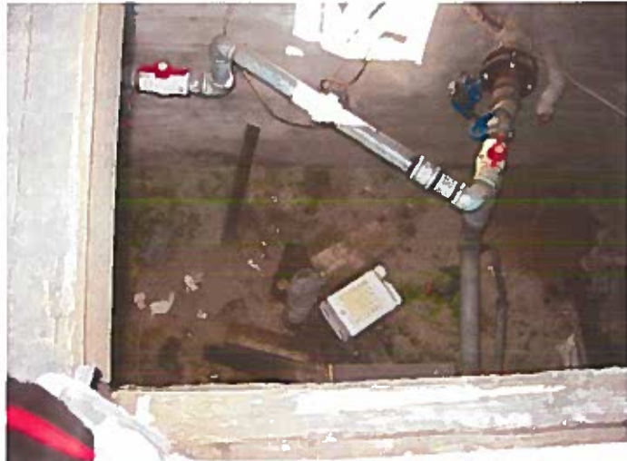
This photo shows the well located on the east side of the office complex and packing plant. GPS reading 2274778 and 1378681. This well is not currently plumbed into the system. GPS reading for this well is;
