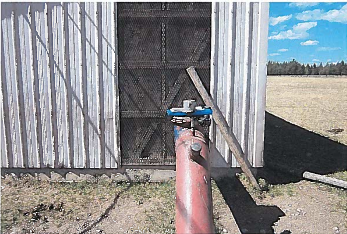
Well in NESE, Sec 15 (Pumphouse & Pipeline) This well not applicable. Appurtenant to 96-7171 (Forfeited)
