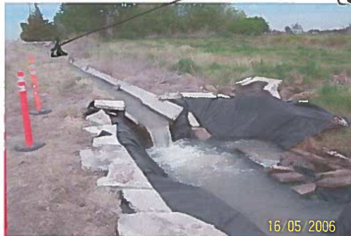
POD: Wastewater 5/16/06 SH
