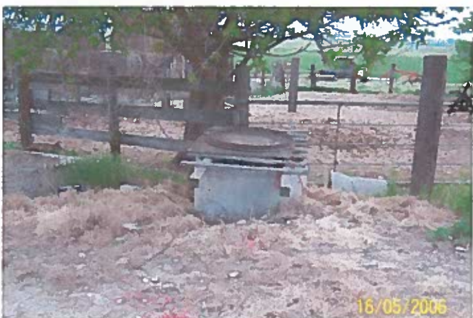
collection/control valves 5/16/06 SH box for 63-21520 + 63-21521
