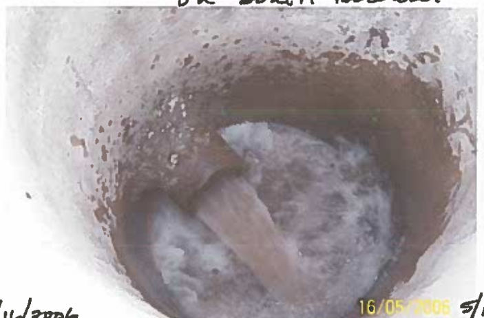
Spring + waste water 8" pipe (full) for 63-21520 + 63-21521
