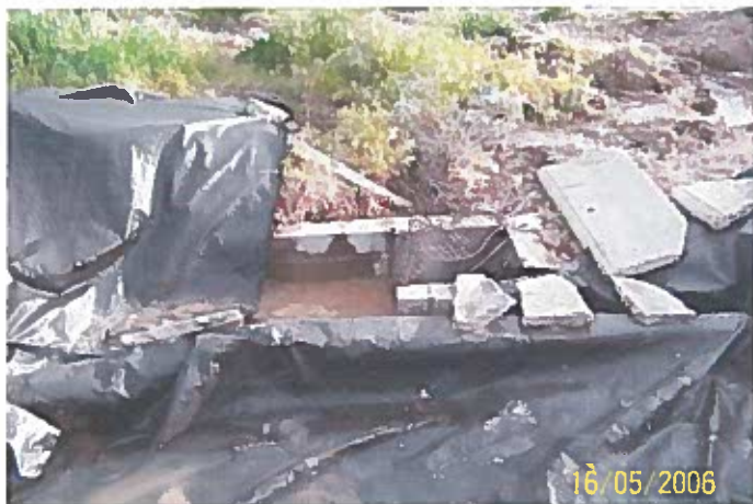
POD: Wastewater 5/16/06 SH for A63-21520 + 21521
