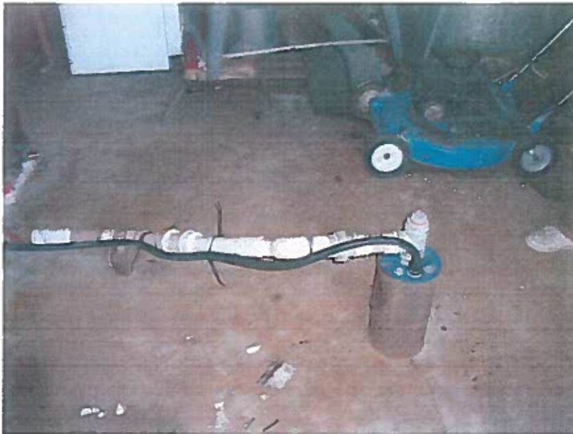
This photo shows the West well.
