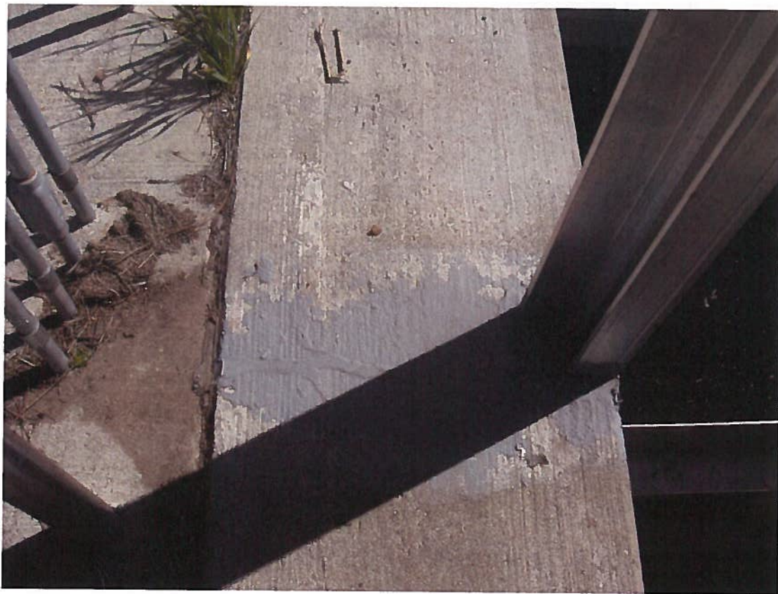
Photo 4 (06/06/2013) - Crack in Right Abutment at Gate Centerline
