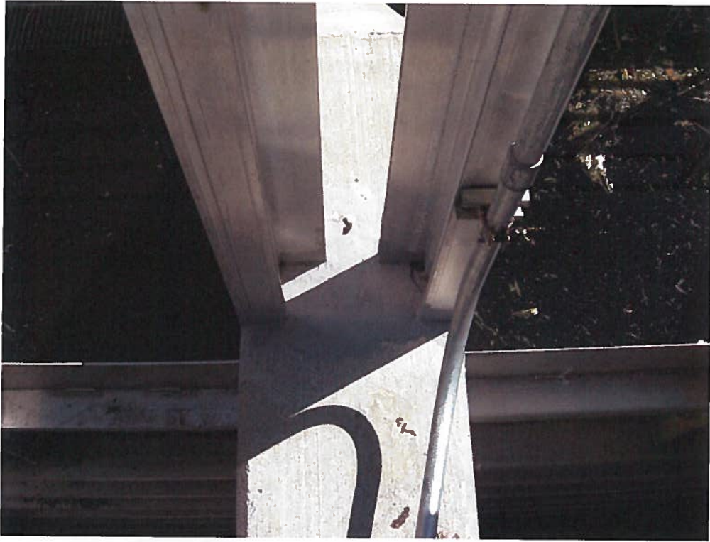
Photo 5 - (06/06/2013) - Right Pier Crack at Gate Centerline
