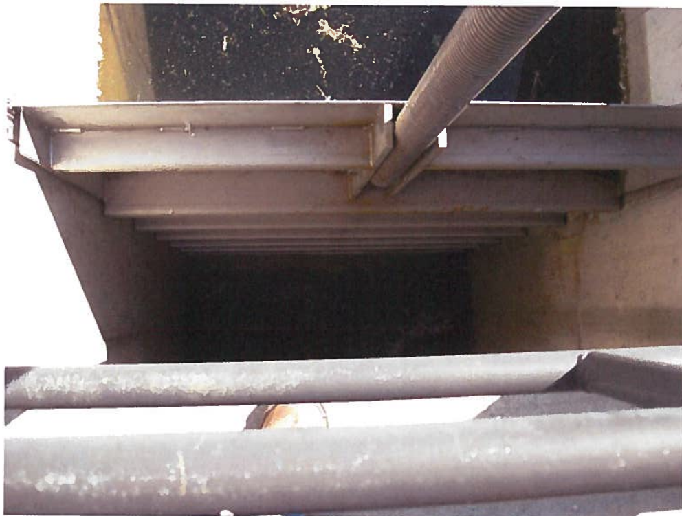
Photo 10 (06/06/2013) - Center Gate Reported Closed, Note Flow at Base
