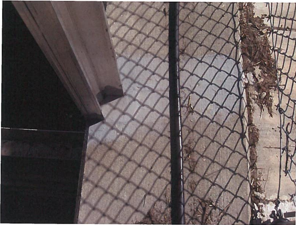
Photo 7 (06/06/2013) - Left Abutment Crack along Gate Centerline
