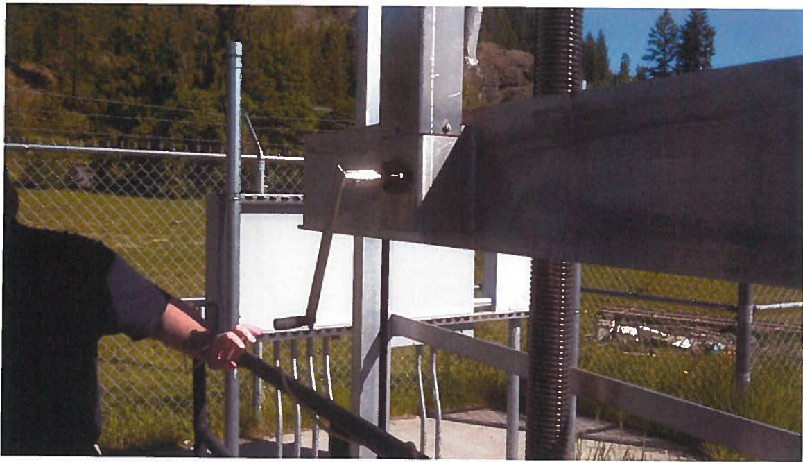
Photo 3 (06/06/2013) - Inoperable Right Gate Mechanism
