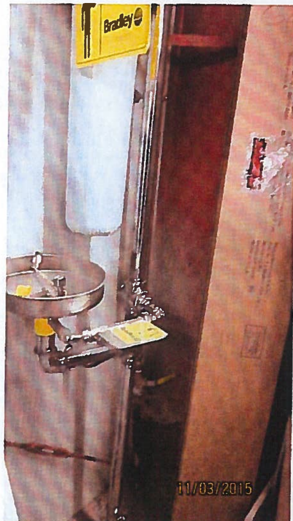
SINK AND FILTRATION SYSTEM IN DECON. UNIT
