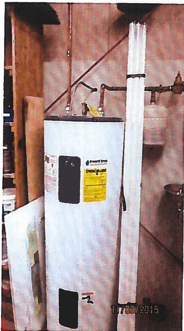
HOT WATER TANK
