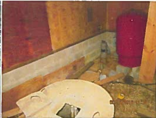
Cistern, pump, and pressure tank (not connected)
