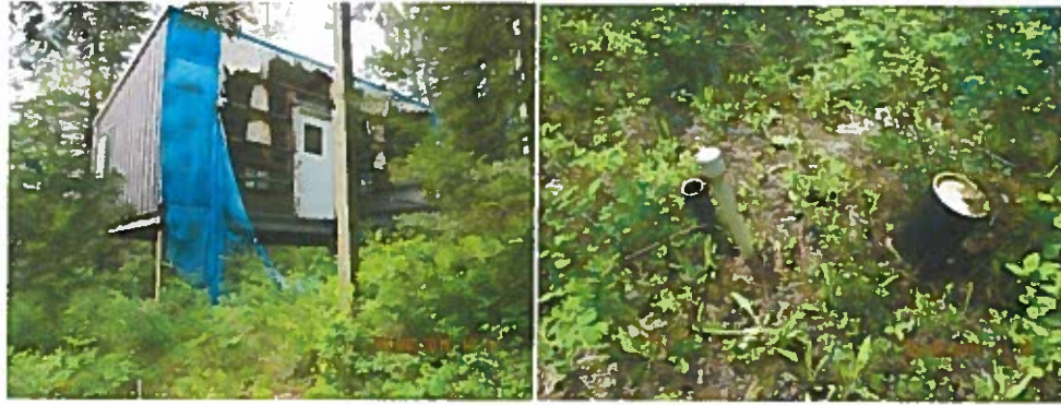
Cabin A – missing wall and pipe stubs. Looks like previous owner intended to expand the cabin out over the stubs eventually.
