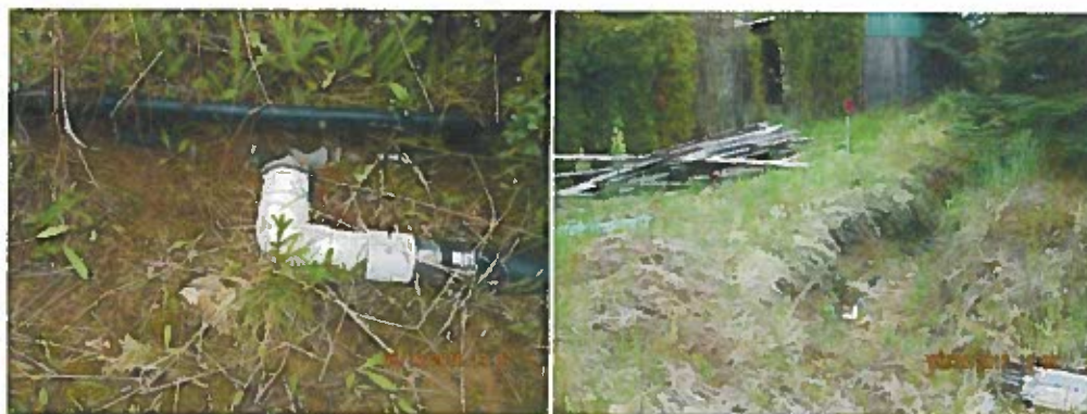
Pipe runs up trench from pond to a T, one side leading to spigot and the other towards a nearby well. Cannot confirm the connection to the well, as the line is buried.
