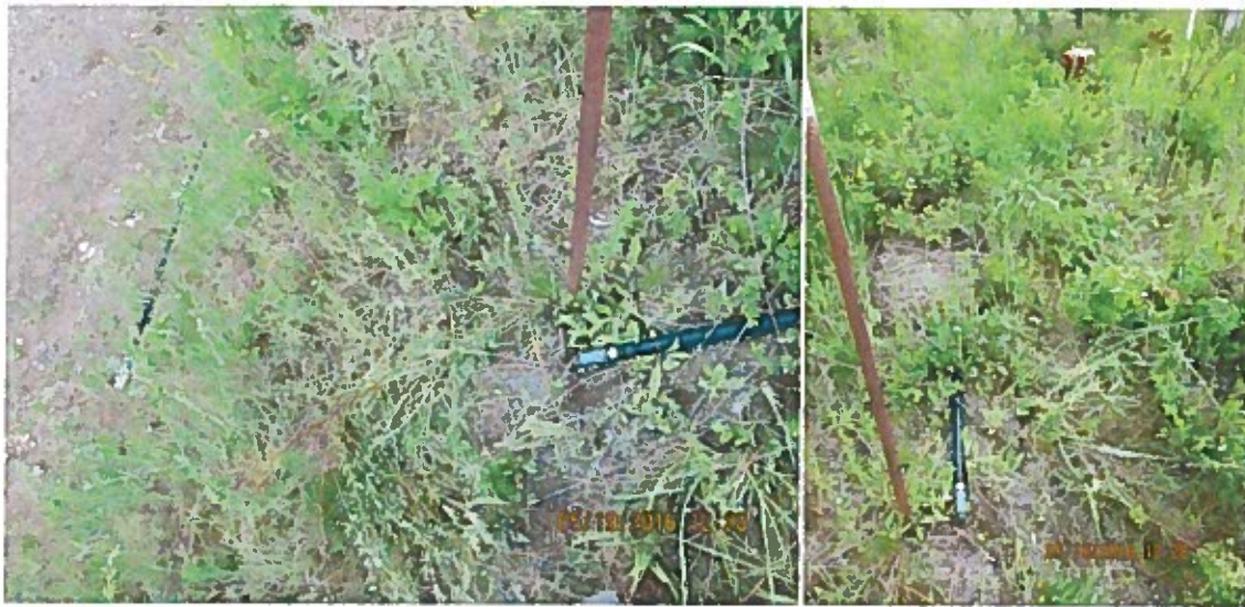
Conduit runs from cistern to connection point at well
