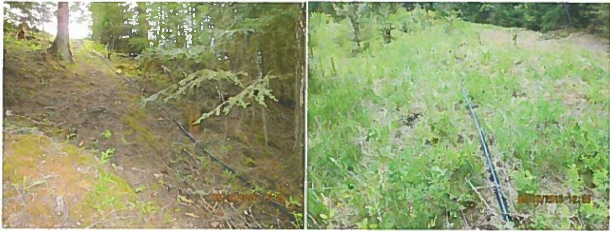
Plastic conduit from cistern up and over hill towards well on south side of home
