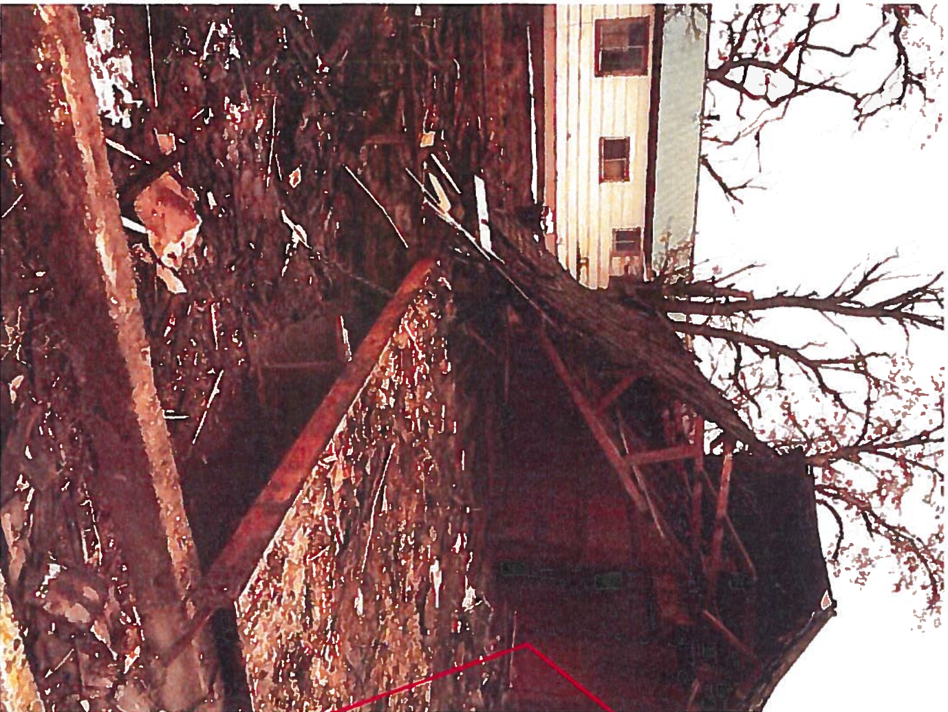
Old homestead being torn down on property. Same red brick that is located at the headbox.
