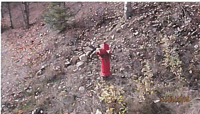
ONE OF TWO HYDRANTS USED FOR FIRE PROTECTION
