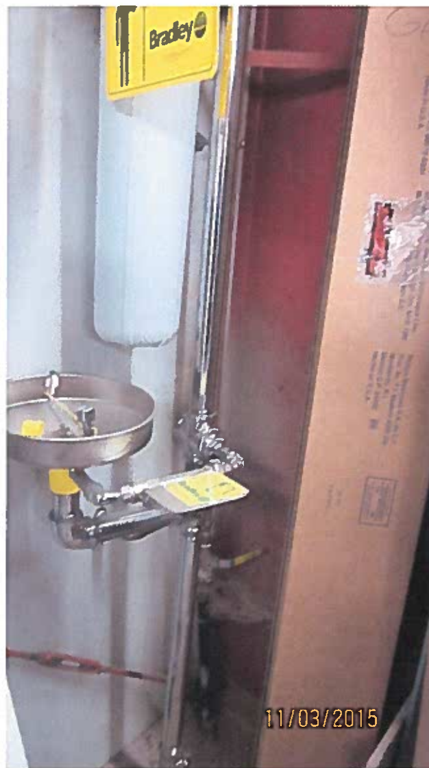
SINK AND FILTRATION SYSTEM IN DECON. UNIT
