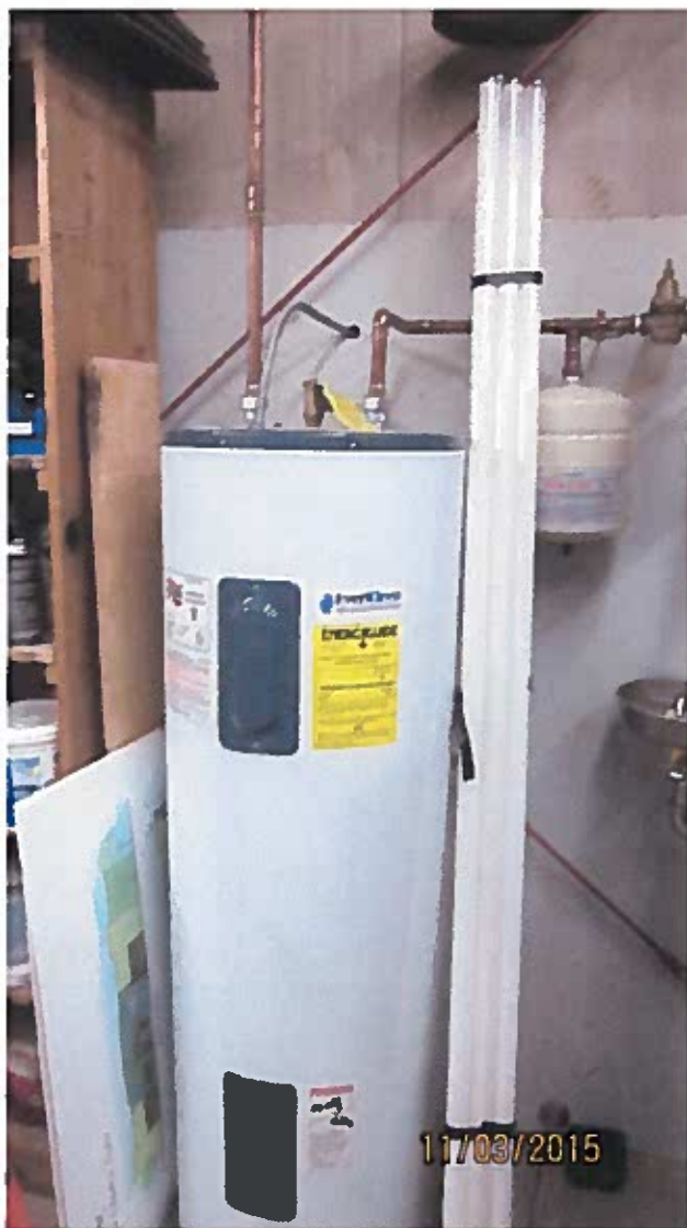
HOT WATER TANK
