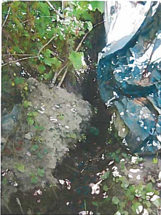
4) Overflow below cistern
