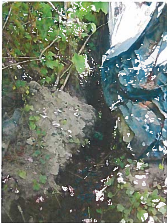
4) Overflow below cistern
