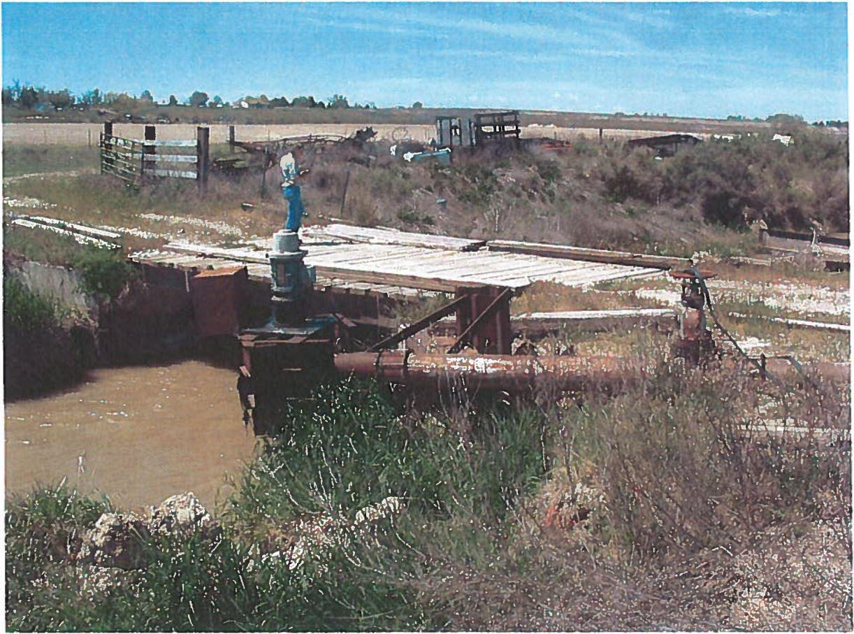
Pump and Discharge Pipe
