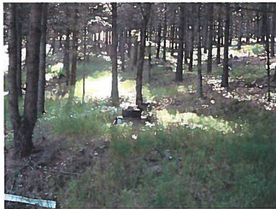
Developed Spring Connected to Water Line
