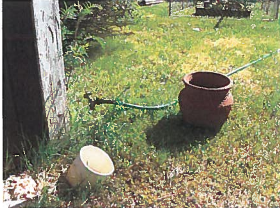
Control Valve Rear Lawn Irrigation Place of Use
