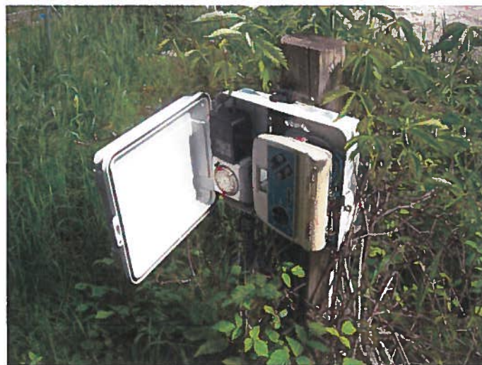
Irrigation Zone Control Box
