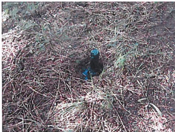
Dripping Sprinkler head
