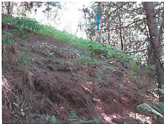
Exposed water line from Creek to POU
