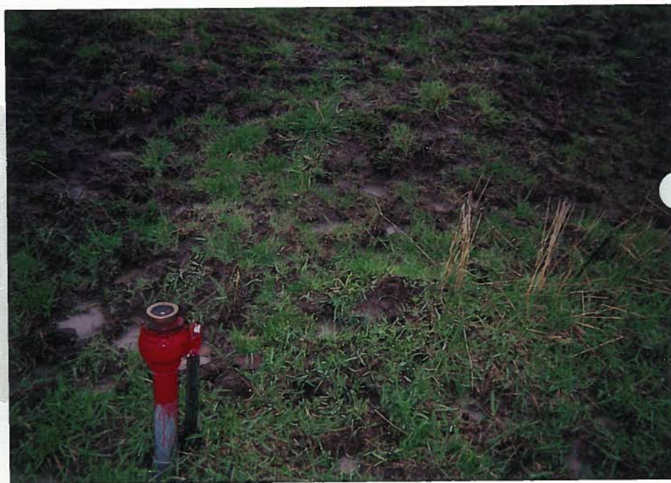
1 of 35 underground sprinkler heads
