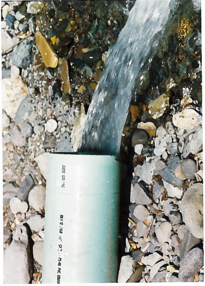
partial discharge from EF-4
