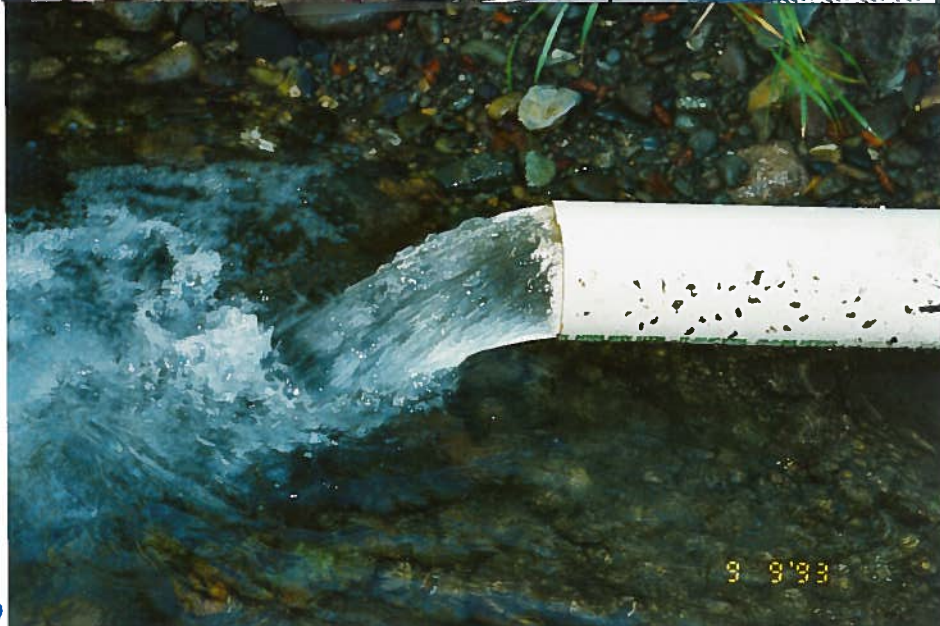
Looking So (upstream) to the Fed. fish trap over the discharge pipe. 9 32 AM.
