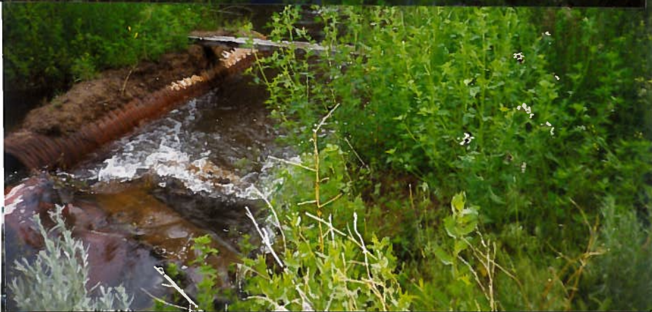
Culvert in Lowline Canal Channel to form pumping pool (Washed out)
