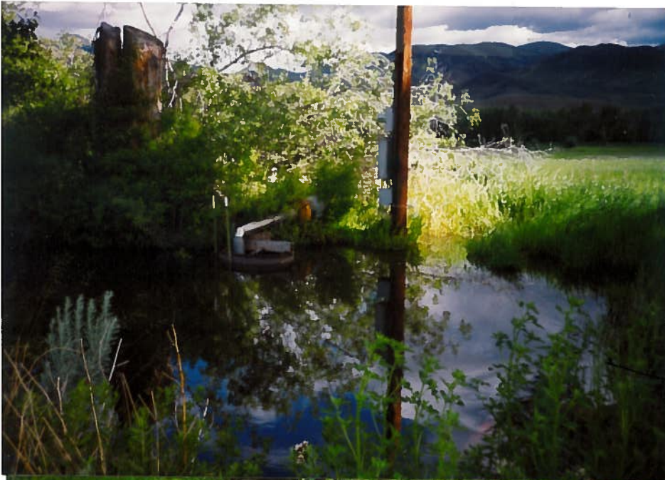
Delbert Hughes Pump Station - from Lowline Canal to Sprinklers 25 HP Centrifugal Pump
