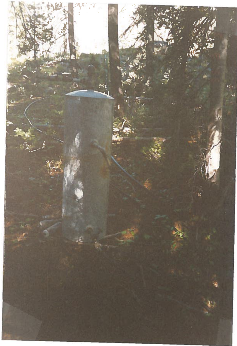
View of FILTER System.
