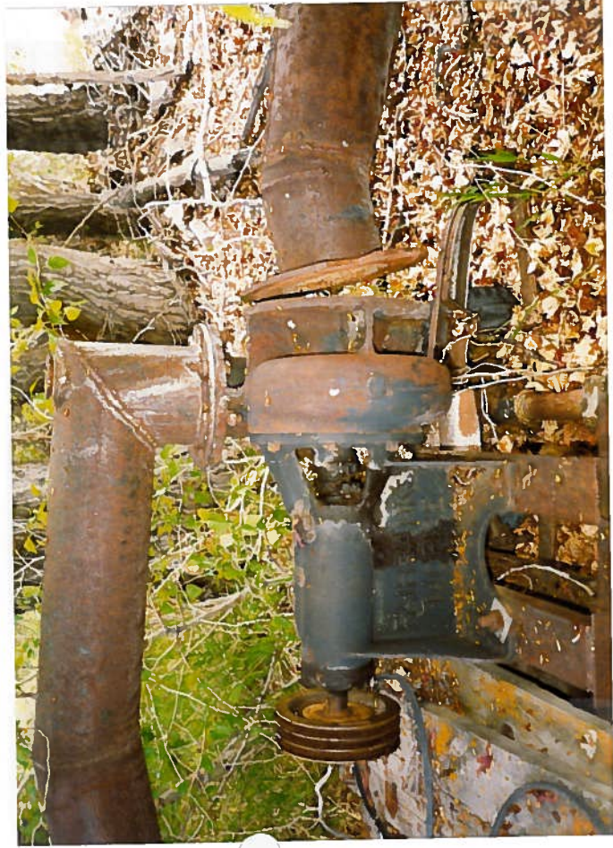
Pump is unusable.
