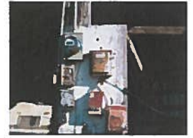
POWER FOR PUMP
