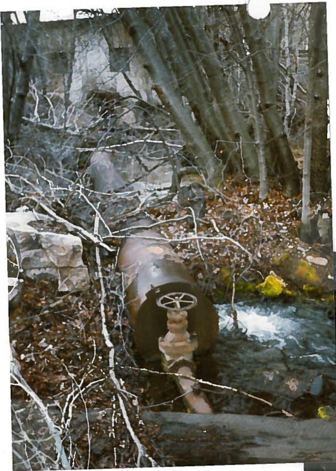
DIVERSION SET UP FROM POWER PLANT ON KINNIKINIC CREEK.
