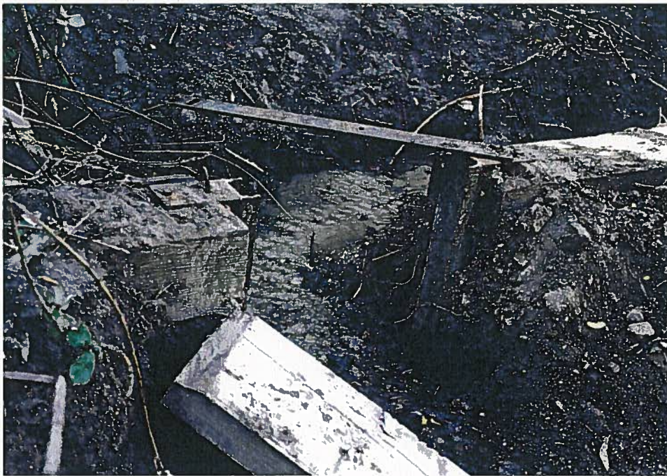
Figure 12. Photographs of the Lower Weir Diversion (Diversion #2) Upper photograph is an April 28, 2005 picture showing the entire Crane Creek flow left in the main channel. CCCC's head gate (extreme right) is closed and no flow is impounded or diverted. Lower view is an October 16, 2004 photograph which shows all of the natural creek being diverted through the CCCC head gate. Lockable stock is visible on head gate. The dimensions and works are described elsewhere in this report and located on Figure 1.
