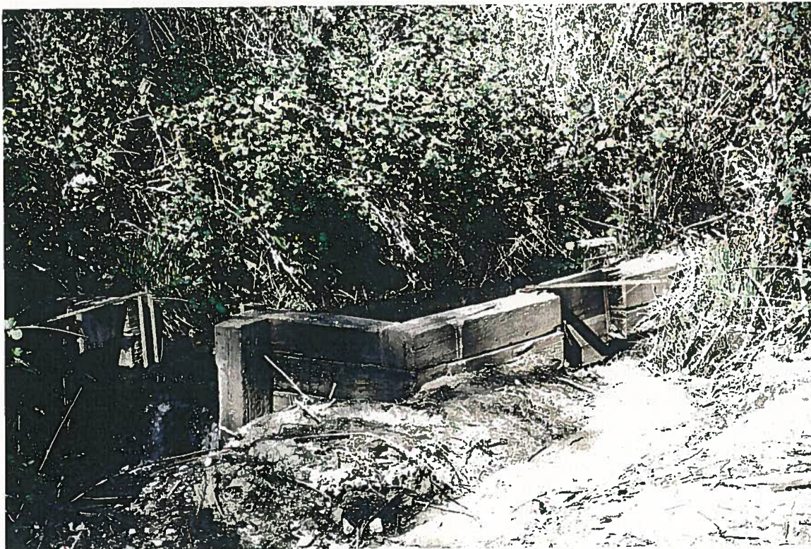
Figure 14. April 28, 2005 photographs of the Crane Creek Country Club's Upper and Lower Weir Diversions on Crane Creek. The dimensions, flow conditions, and works are described elsewhere in this report and located on Figure 1.
