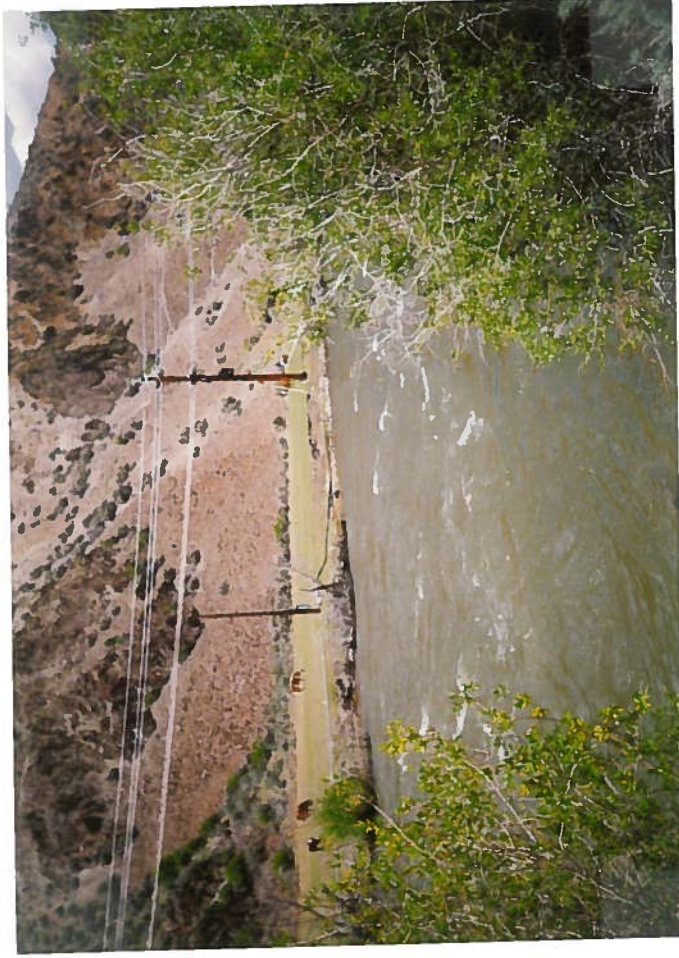
↑ Pump in river.
