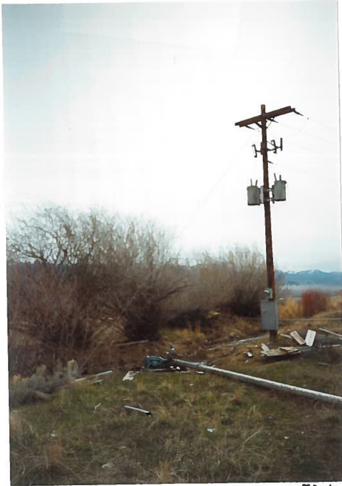
View of DuBois pump station along the High Line Canal. Looking SE 40 HP pump Centrifugal pump 6" inlet, 4" to 8" (expanded) outlet
