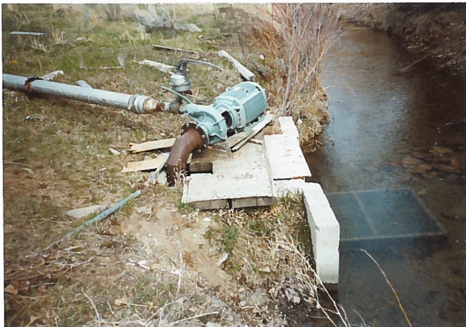
As above showing close view of pump and intake structure.
