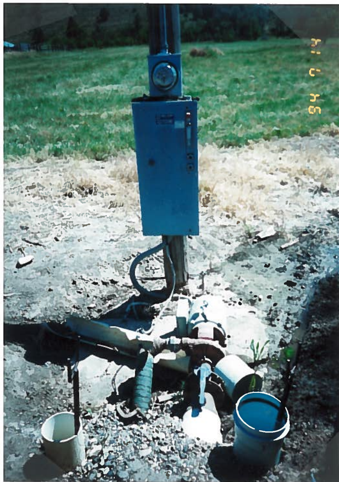
Pump @ STANGER DITCH PIPELINE.
