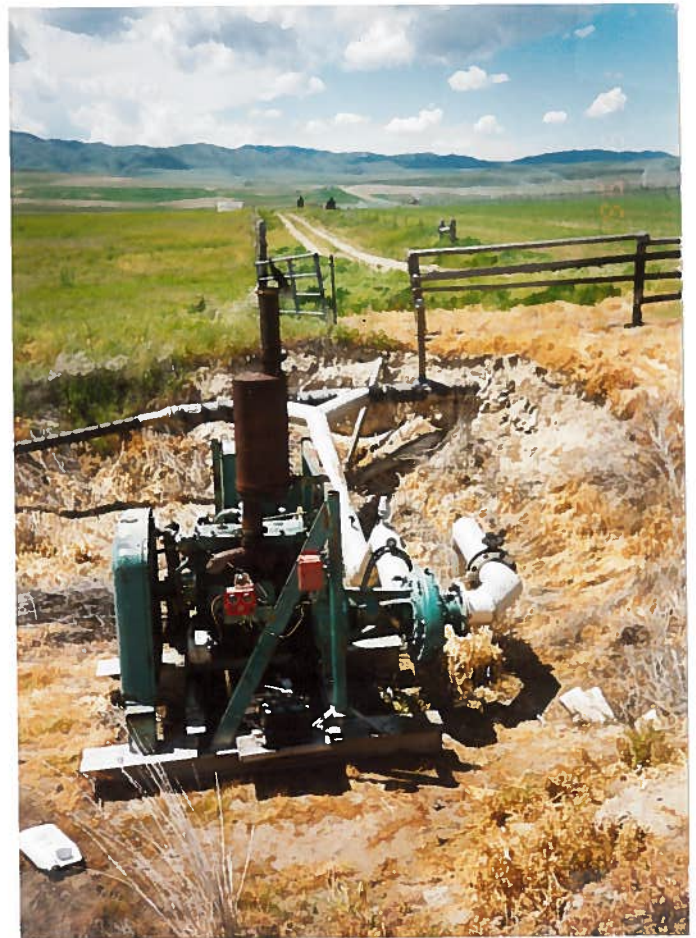
Diesel Pump system. View West
