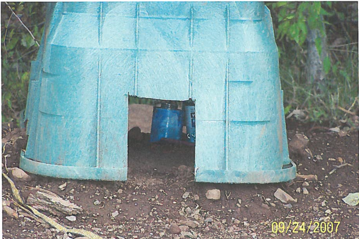
Control Valve under cover
