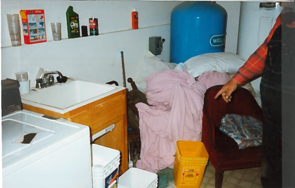
New well located inside laundry room under floor in motel.
