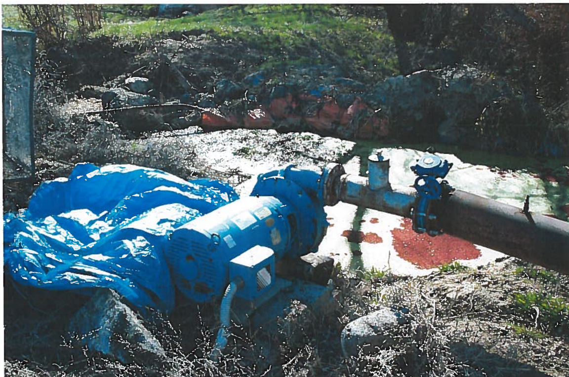
Sump & Irrigation Pump On Birch Creek, Claim 37-797 By J E Stanton 3-9-05
