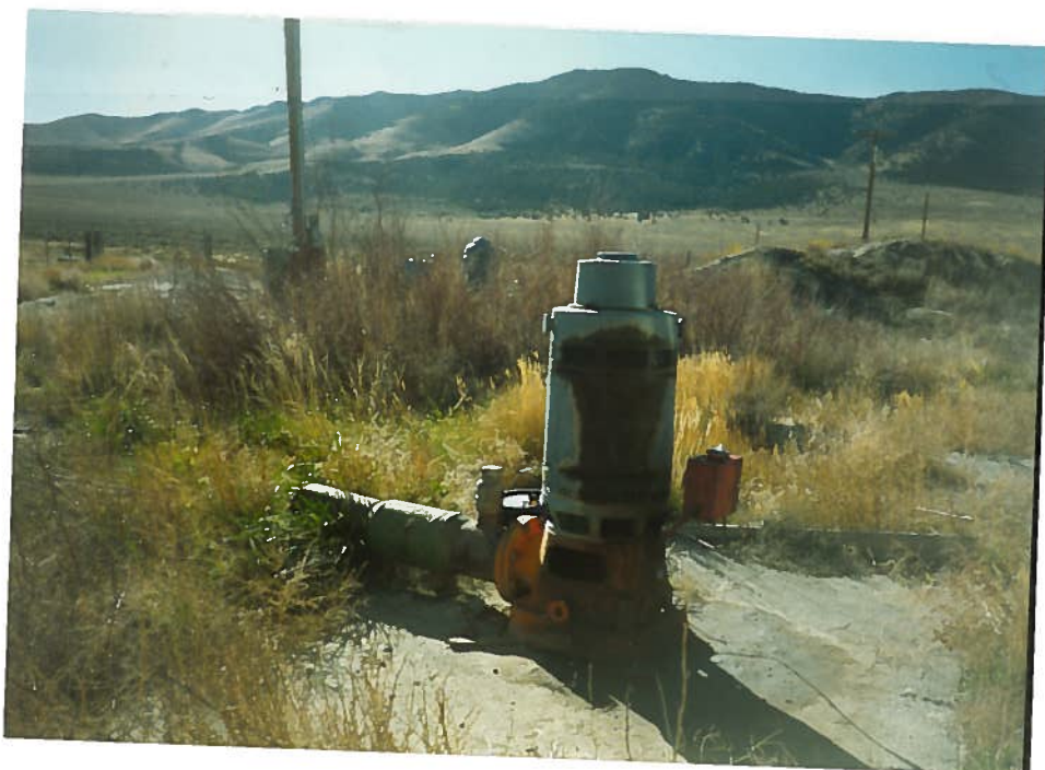
Well #2 T12S, R26E, Sec. 11 SWSWSW 100 h.p. motor (closer to house)
