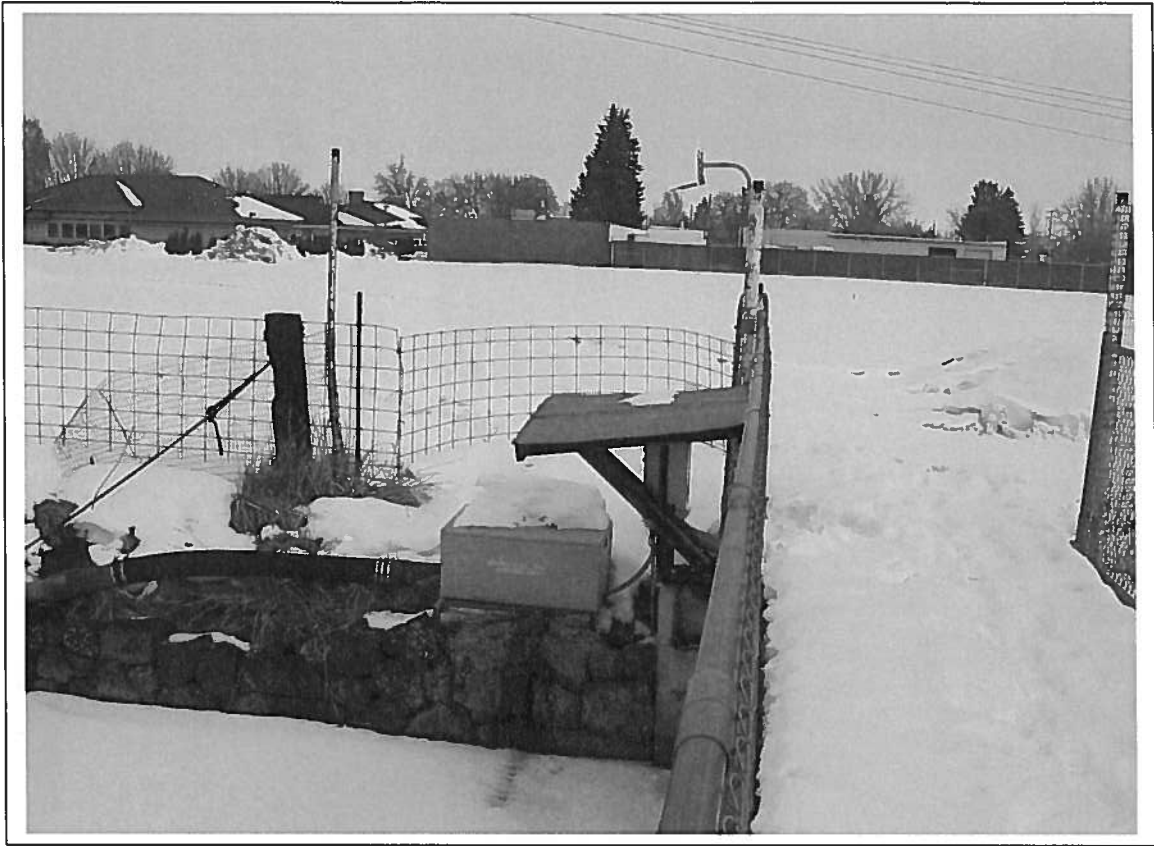
School Pump 01/28/2004 Tag No. A0011706
