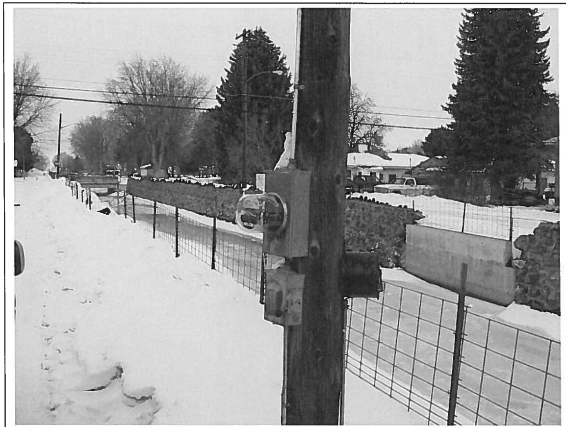
Main Street Pump 96-P 01/28/2004 Tag No. A0011707
