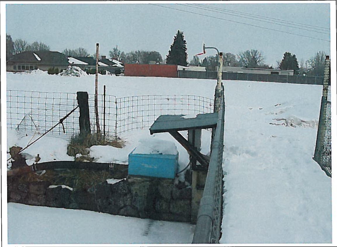
School Pump 01/28/2004 Tag No. A0011706
