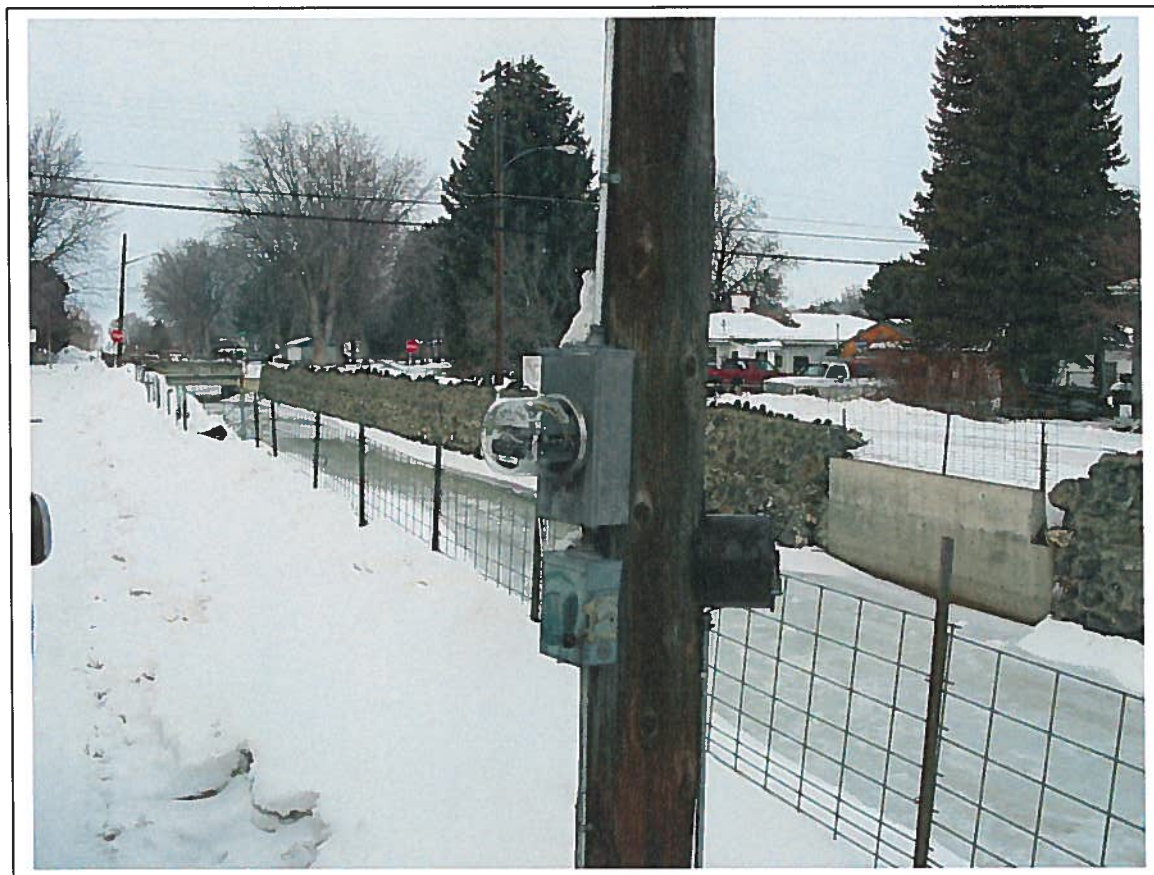
Main Street Pump 96-P 01/28/2004 Tag No. A0011707
