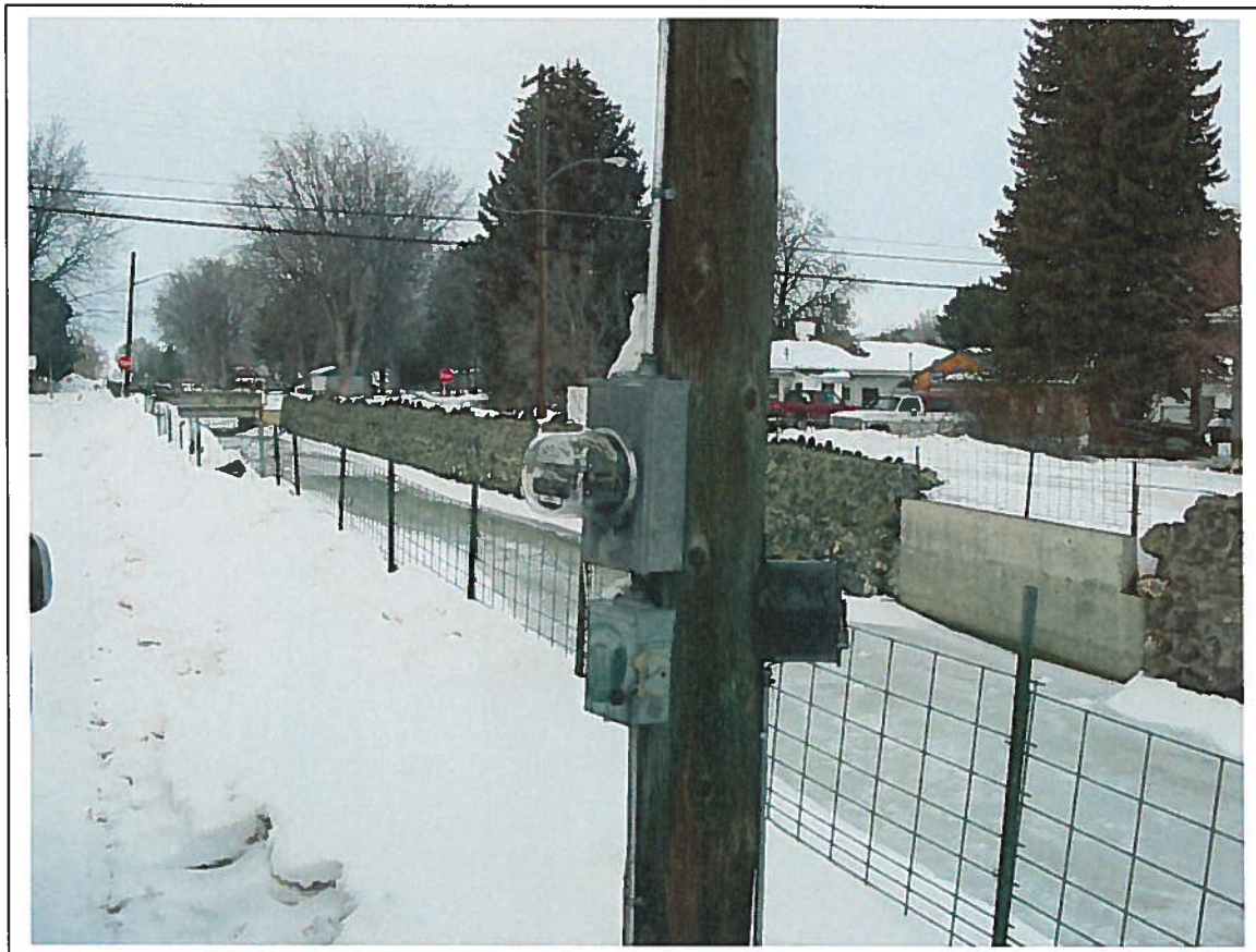
Main Street Pump 96-P 01/28/2004
