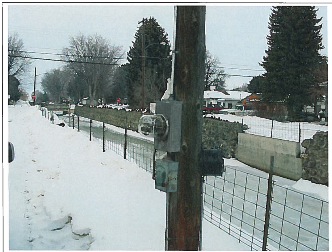
Main Street Pump 96-P 01/28/2004
