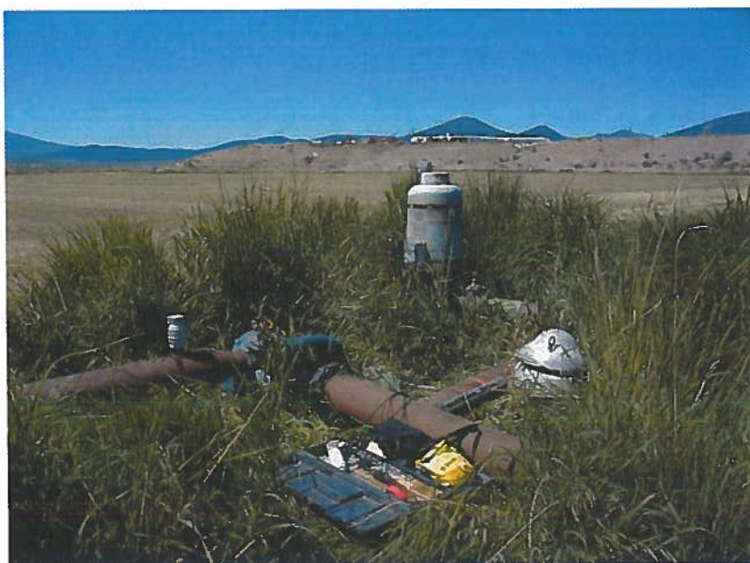
14. Kent Durfee pump in section 12. T16S R24E South pump.
