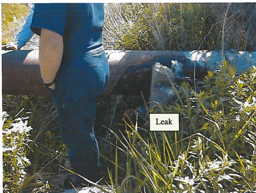
12. Close-up of the Bruce Durfee's leaky pipe.
