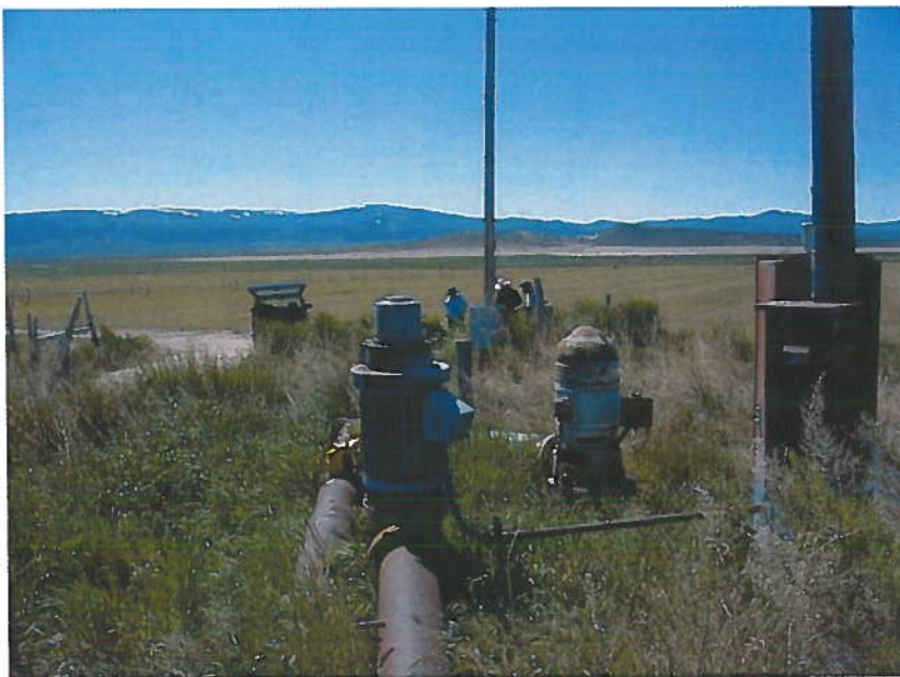
18. Looking south from the Kent Durfee booster pump at the POU.
