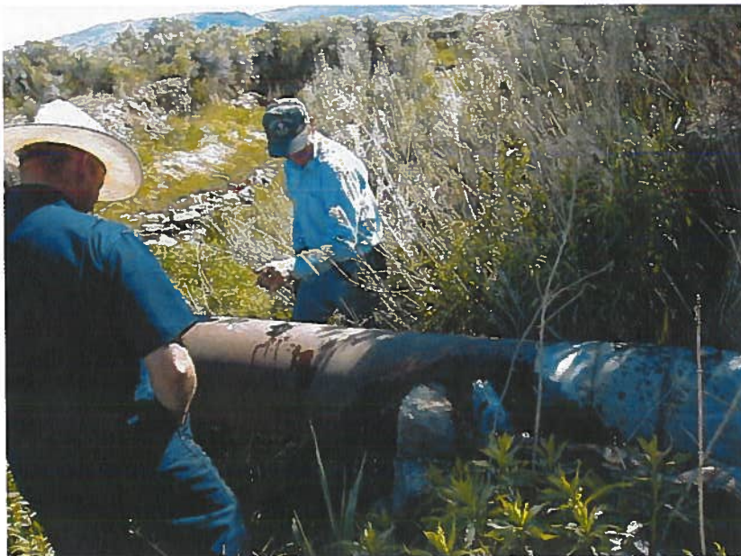
11. Bruce Durfee's pipe from T16S R24E section 23 POD. The leaky pipe returns water to the Raft River.
