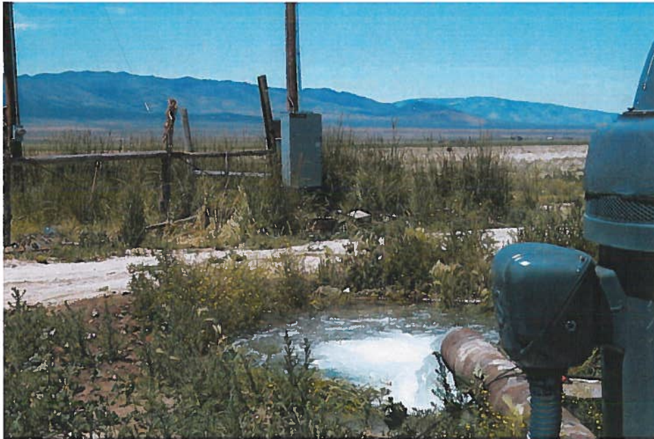
Figure 3: Looking NW North from Gardner's new pump to the old abandoned well. This well was abandoned because a tool was dropped down the well. The old well is located in front of the power pole.
