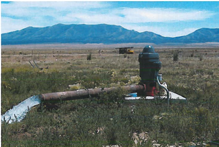
Figure 2: US Electric 125-hp motor. Serial number R2020949. GPS file name: T-62119A. Pump: Layne and Bowler, Serial number LP99061/12T. Flow was measured with the Polysonic flow meter at an average of 1573 gpm or 3.51 cfs.
