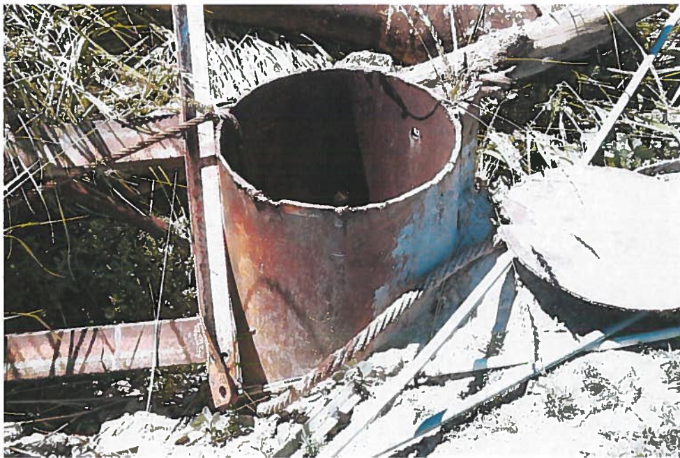
Figure 4: Close up of the abandoned well. The water level was measured on the south side of the well casing. The level at the top of the casing was 6 feet 3 inches. The casing was marked with the point of measurement and the depth. GPS file name GARDNOLD.
