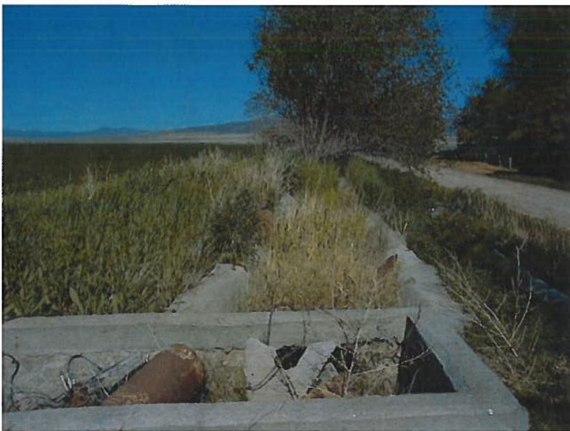
Figure 7. Old concrete ditch system.
