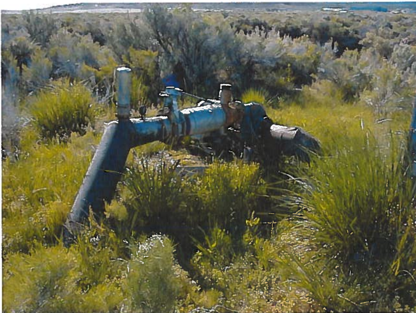
6. Close-up of Kent Durfee's booster pump to pivot in section 14.
