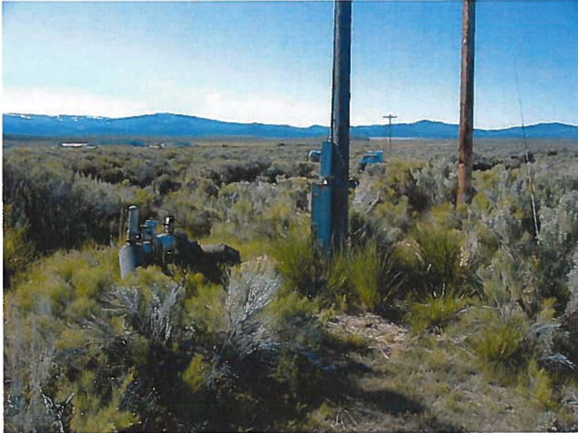
5. Kent Durfee's booster pump to pivot in section 14.
