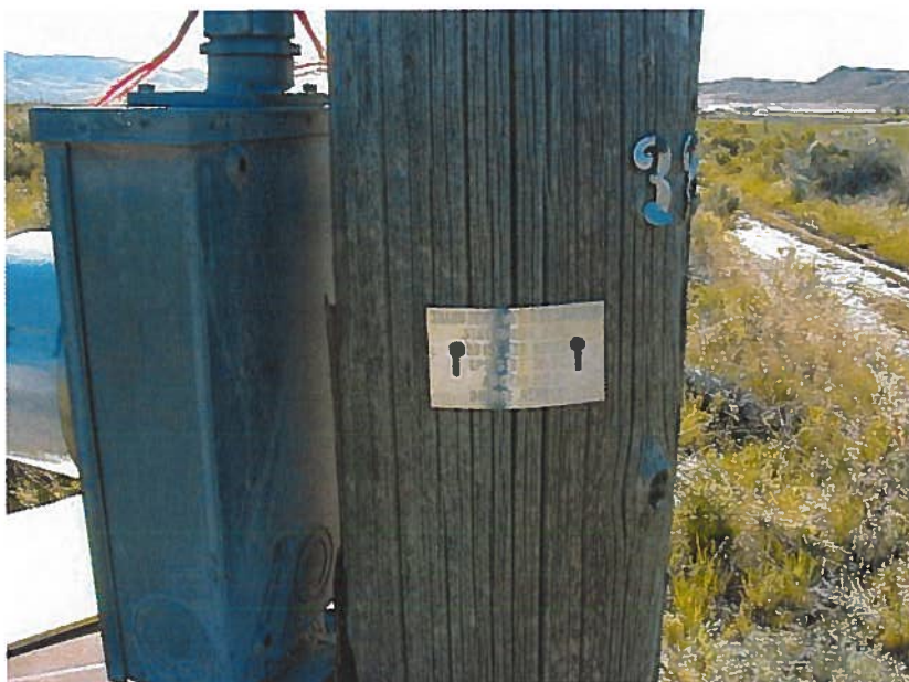
1. Site tag at Kent Durfee's well. T16S R24E Section 14 A0008915
