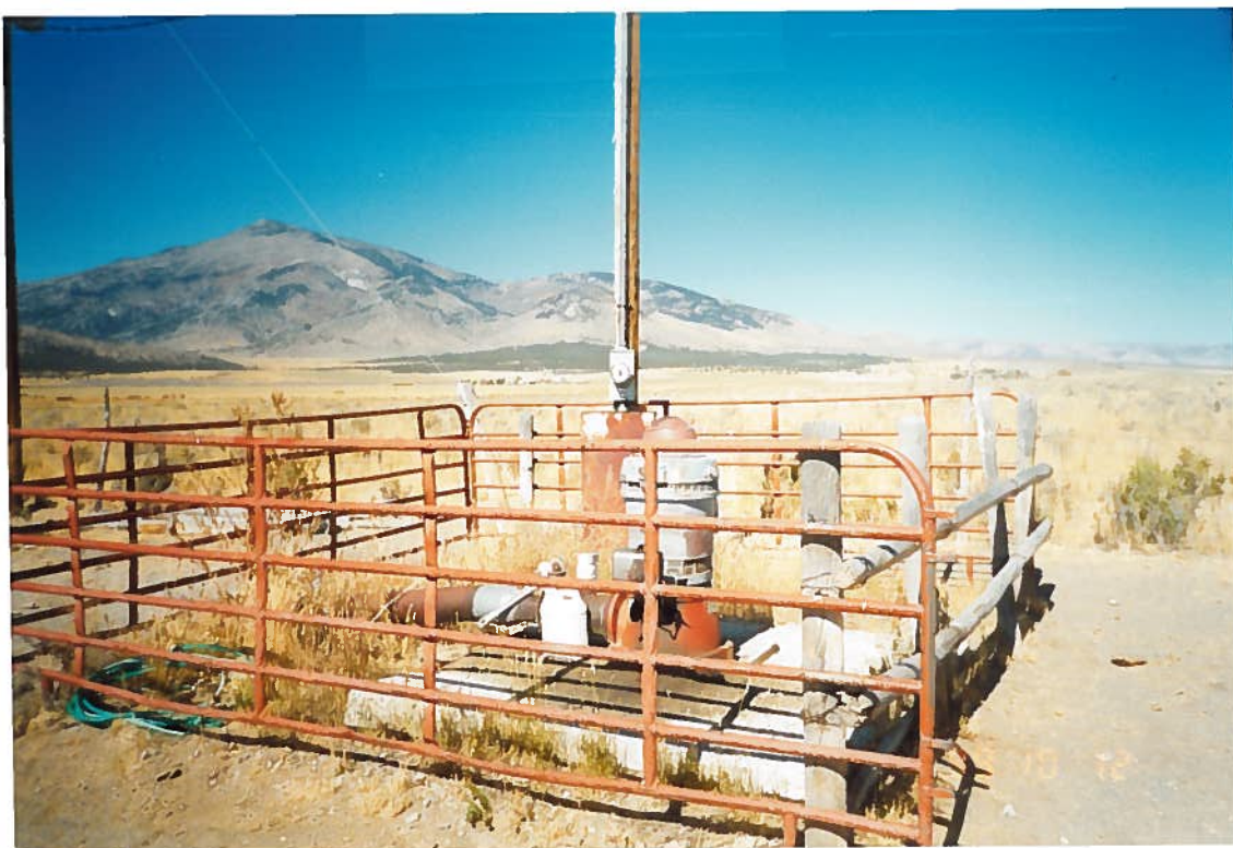
Well in NWSE Section 18 R101219A TAG ON power pole. A0004846 GPS
