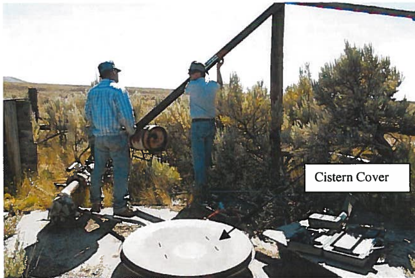
Figure 3. Scott King applying the transducers to the discharge pipe in preparation for measuring the flow. The Fuji Flow meter was used to measure the flow.
