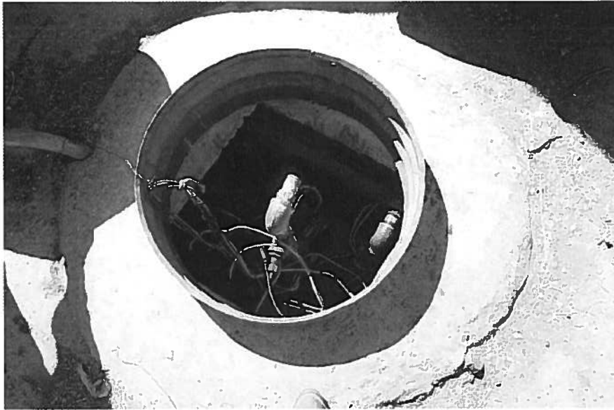
Figure 5. Cistern used to house the submersible stock water pumps.
