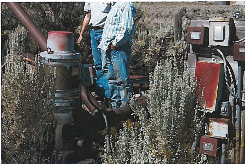
Figure 2. 15 hp U.S. Electrical Motor and Layne & Bowler pump assembly for C Bar Cattle Company.
