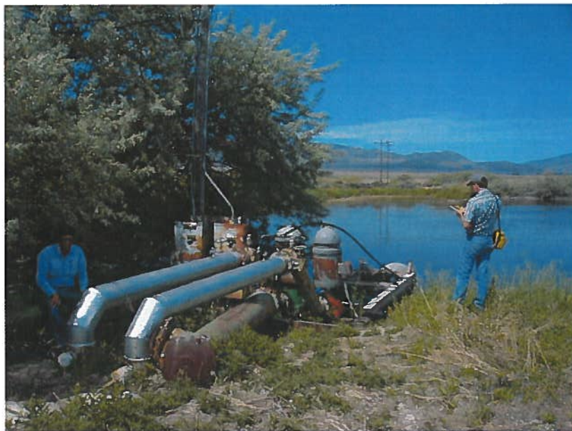
Figure 4. C Bar pond. 2-75 hp pond pumps are located on the eastside of the pond. North or lower pond. GPS file name 19033AAA, pole number 180169.
