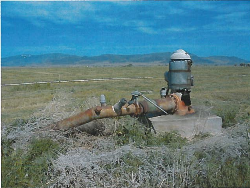
Figure 1. C Bar/Arimo (previously Pierce) U. S. Electric 60 hp motor S/N 1158803. Layne and Bowler Pump s/n 25092 2200 gpm. Power pole # 19043, meter s/n 28065820. T13SR27E Section 30 SESE. GPS file name 19044AAA.
