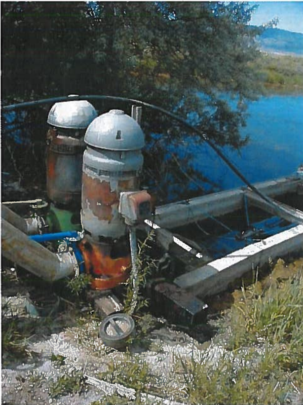
Figure 7. C Bar 2-75 hp pond pumps.
