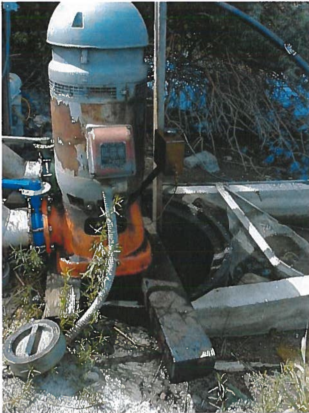
Figure 5. Close-up of the 2-75 hp pond pumps.
