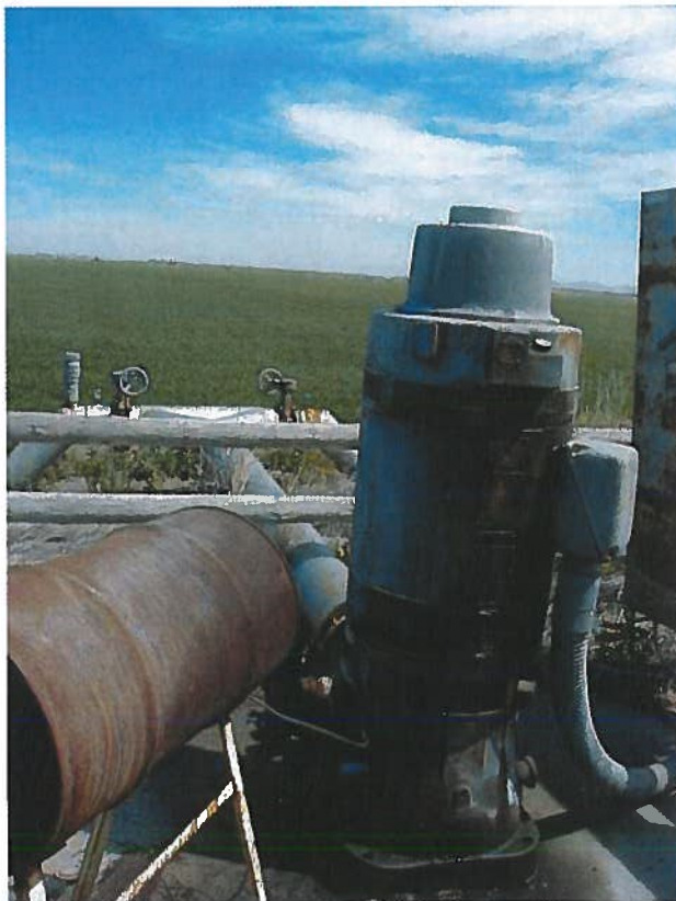
Figure 10. 200 hp well pump meter s/n 95861859. Pressure or discharge to the North pond.
