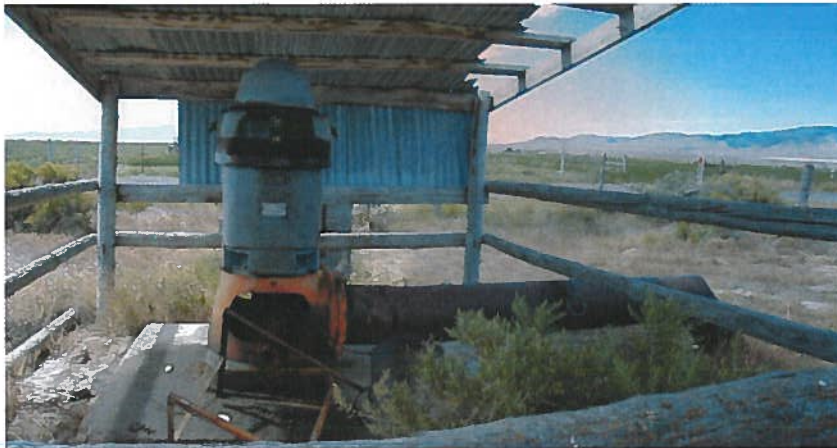
Figure 3. C Bar/Arimo Corp. U. S. Electric 150 hp s/n C2931-00-168. Layne & Bowler Verti-Line pump s/n 23911, 2700 gpm. The pump open discharges into the Raft River, Column and discharge pipe is 12". Power pole number 19066, meter s/n 78830105. GPS file 19033AAA.
