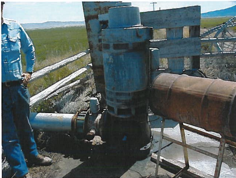
Figure 9. C Bar (Arimo Corp.) U.S. Electric 200 hp motor, s/n DKJ417115. Power pole 19033. GPS file name 19033AAA.
