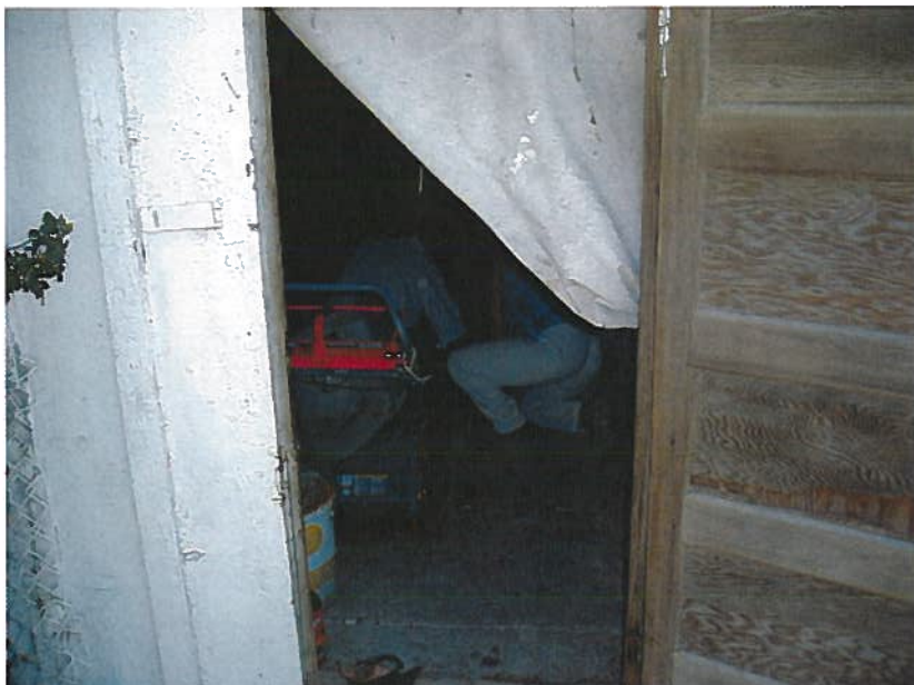
Figure 3. Inside the pump house at the Naf Mercantile. T16S R27E S27.
