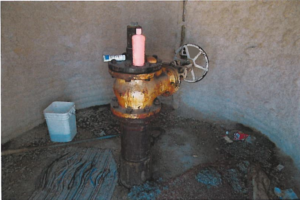
Figure 3 Inside the well house
