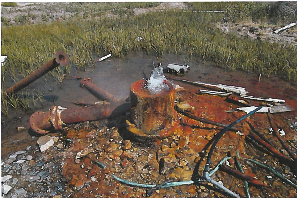
Figure 4 Abandoned uncontrolled Geothermal Well at Gary Crook's site.
