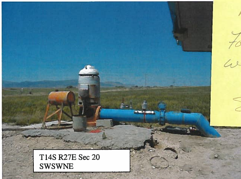
Figure 1. 175 hp well pump. Looking north. GPS file A0007911. & Site Tag
