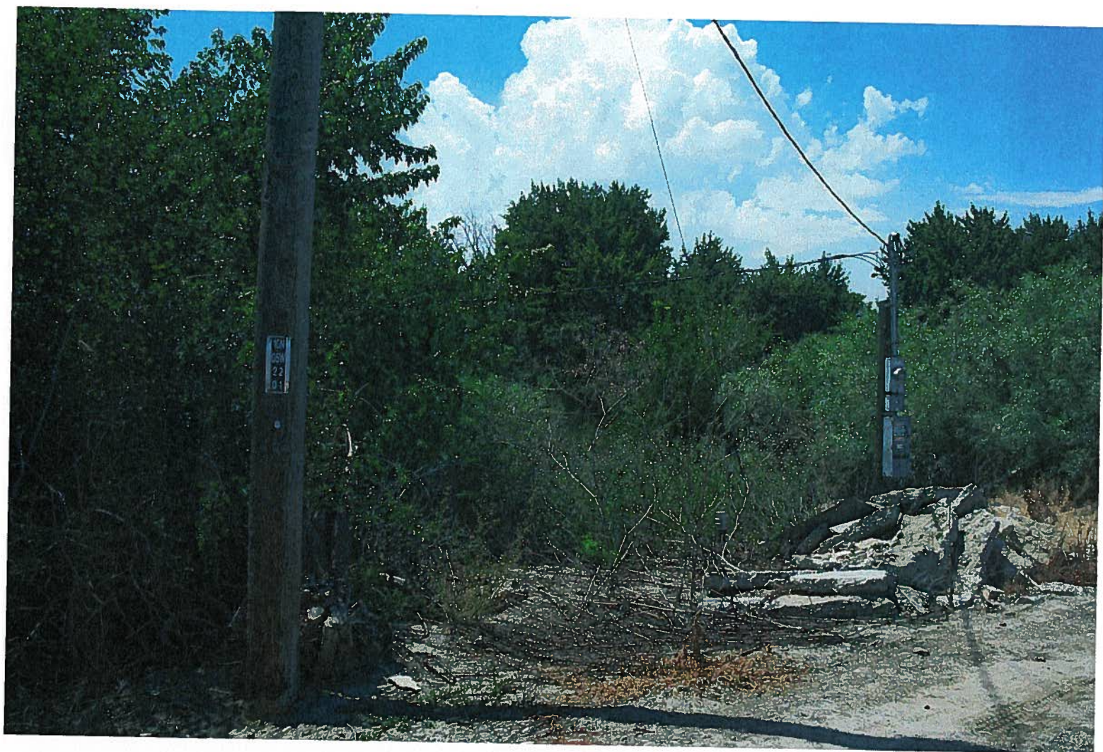
3-401b Power Service Pole 7-29-05
