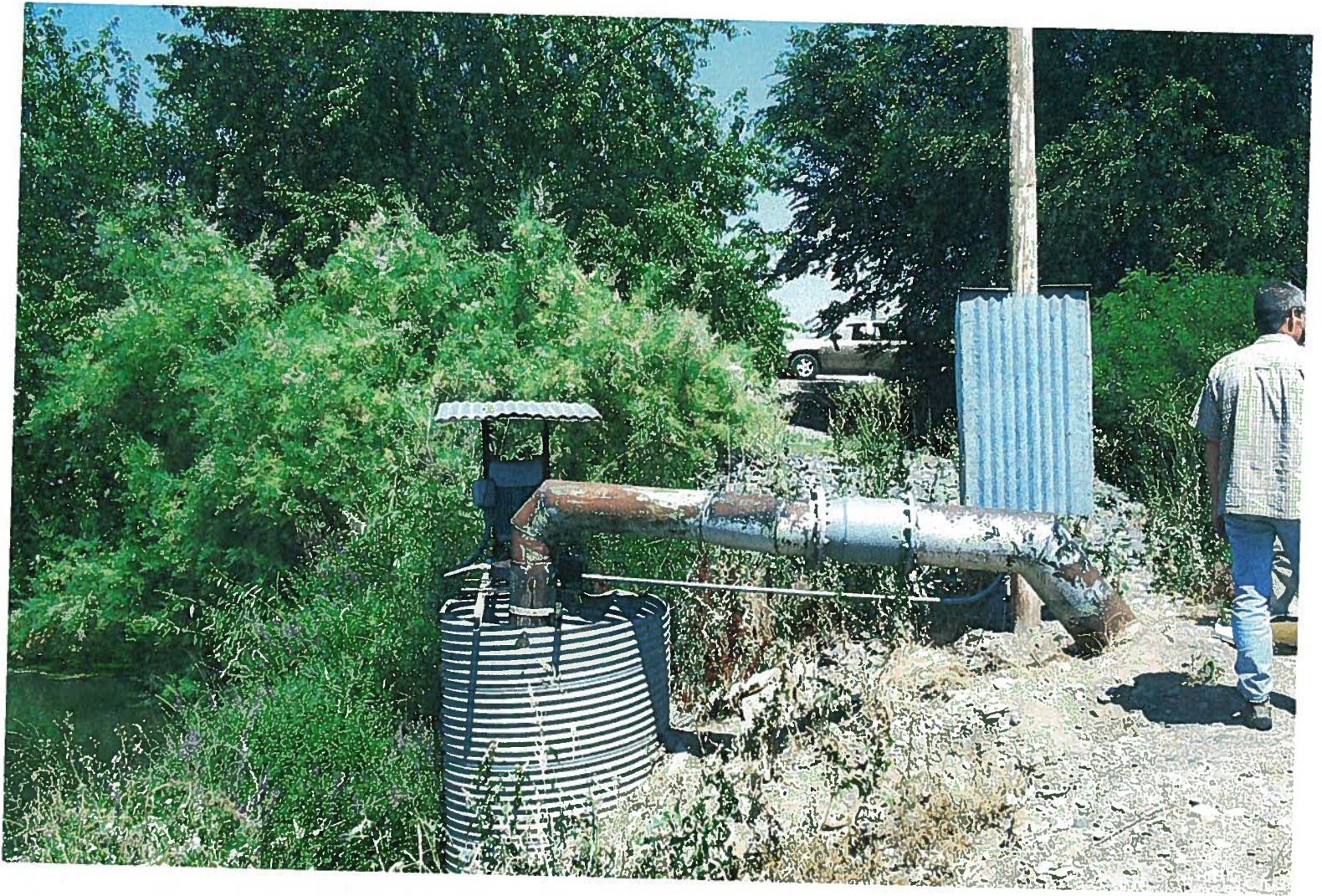
3-4016 Pump for East Field 7-29-05
