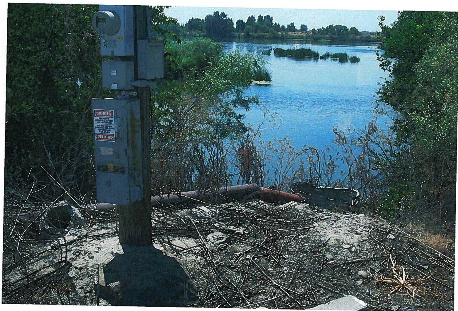
3-4016 Pump Platform for West Field 7-29-05
