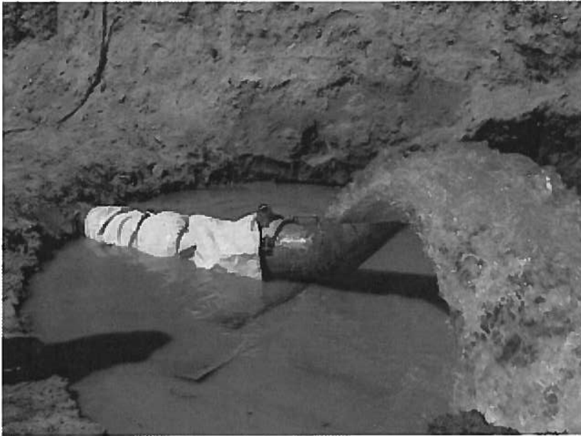
Figure 7. Flow measured at 3477 gpm by Jerry Udy.
